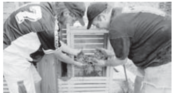
The mix was delivered to the walls with wheel barrow. Daniel Thomas (right), of Hammer & Hand (general contractors) and coworker placing mix in walls.
