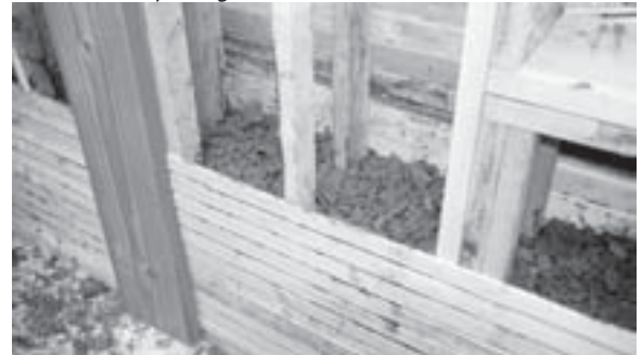
The mix was placed in a 12" cavity made up of 2x4 light framing and wooden laths. Over 90 feet of wall was filled during the 5 day workshop. The crew completed the remaining 100' of wall infill in an additional five days.
