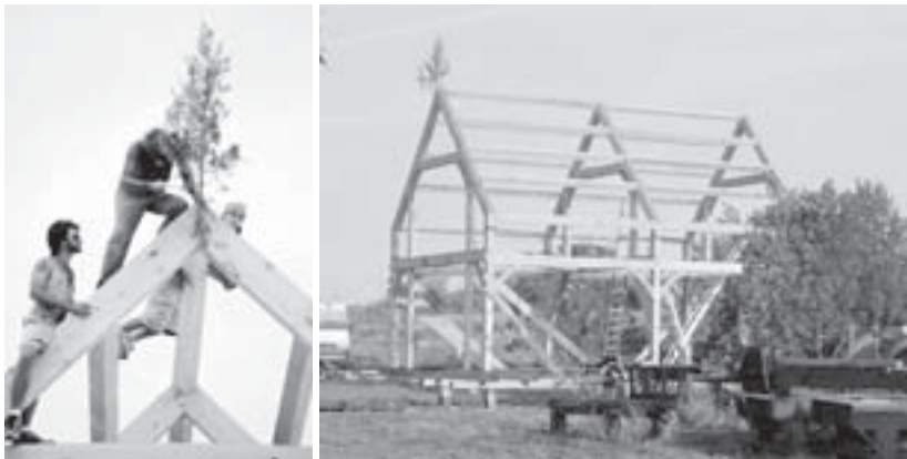
Aloysius Weasel Bear using chain mortiser for the first time; Tom Cook nailing roof tree with Jayson and Nefu; Completed frame with Belsaw mill in foreground.
