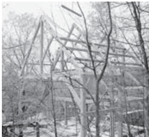
White and red oak timber frame cut in the Airville, PA, Workshop, April, 2002.
